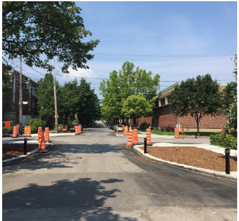
Figure 22: Laurier and Des Erables Curb Extension (under construction), Montreal, QC; Credit: Julia Malmo-Laycock
